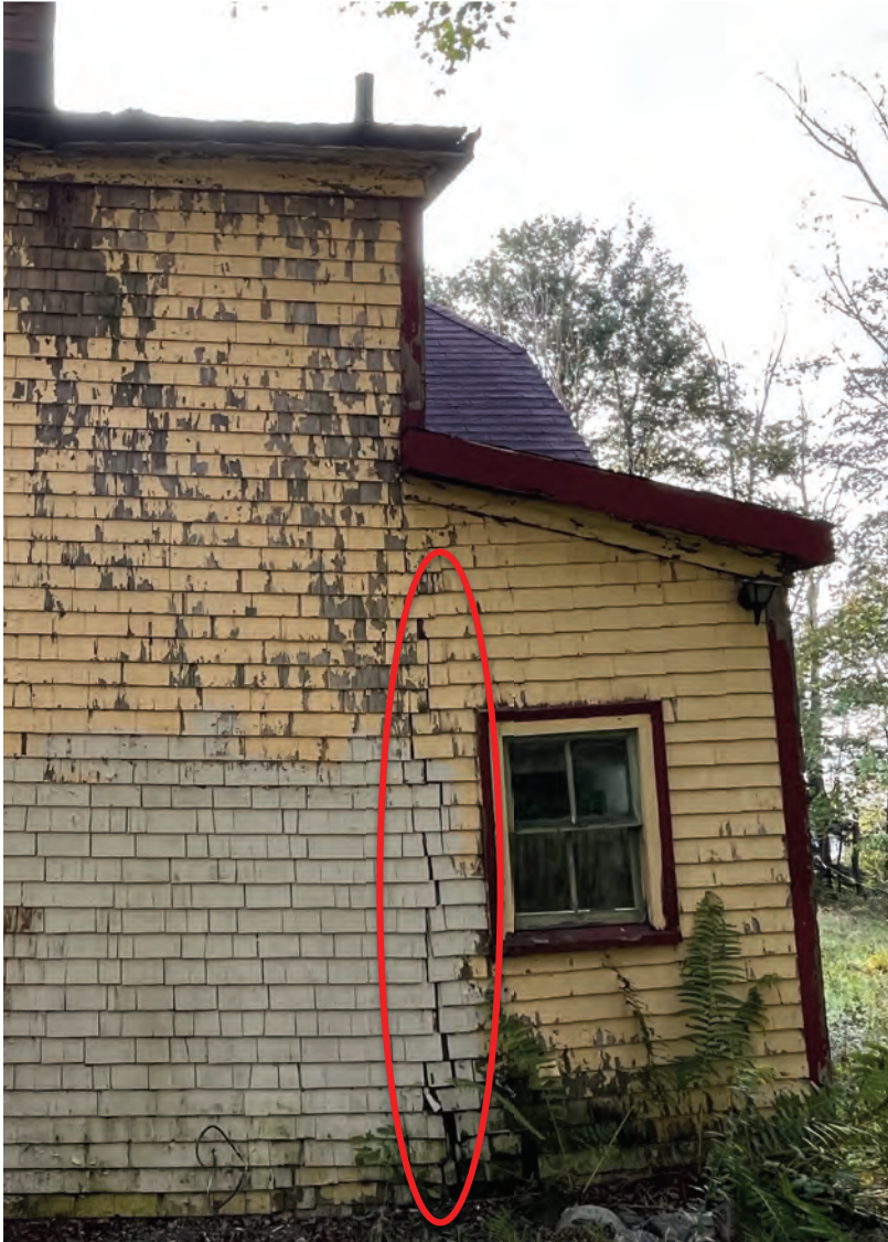
Figure 25: Separation occurring in the rear wall face as a result of settling.
