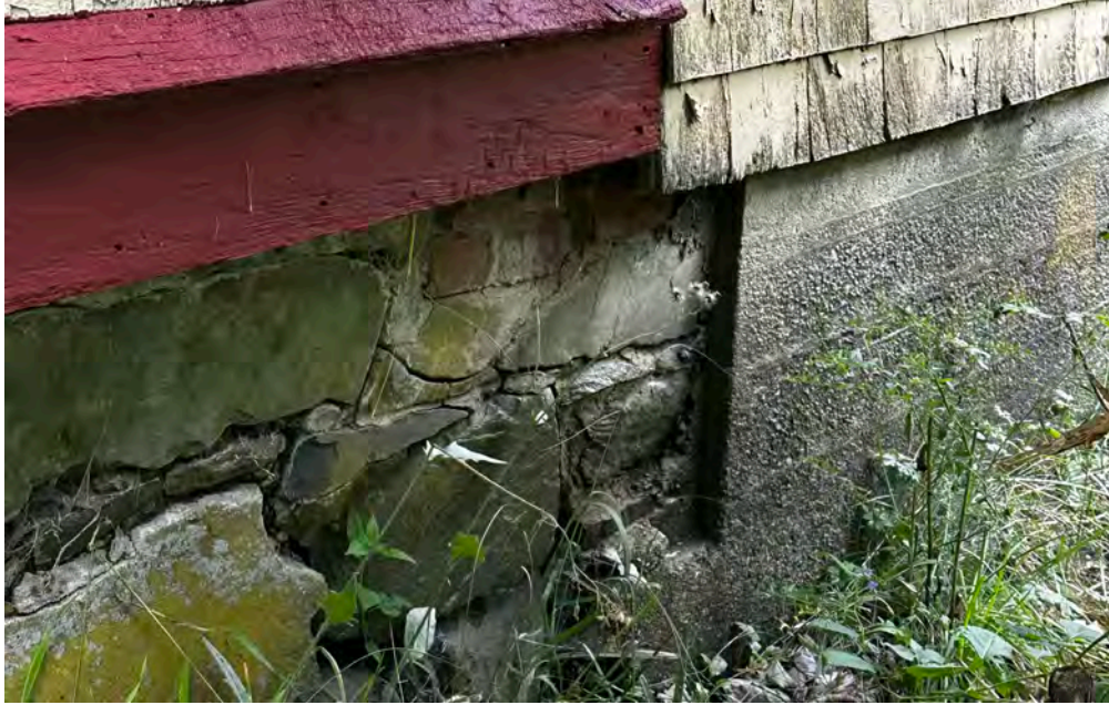
Figure 11: Close up picture of foundation difference along Red Gable's south elevation (Staff photo, July 17th, 2024)
