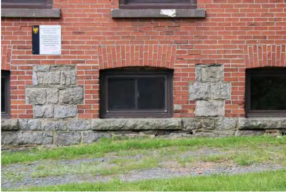
Photo 14: Stone foundation and cut stone inclusions on the east façade, looking west
