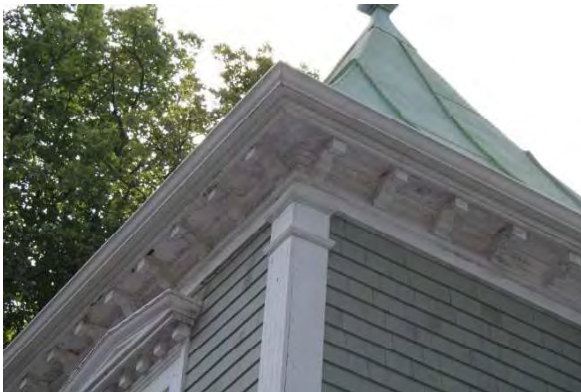
Photo 10: Wood soffits, brackets, and corner pilasters on the front façade, looking southeast
