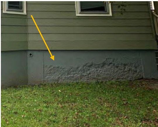
Photo 14: Visually distinct concrete section at northeast corner of front façade (denoted by arrow), looking west.
