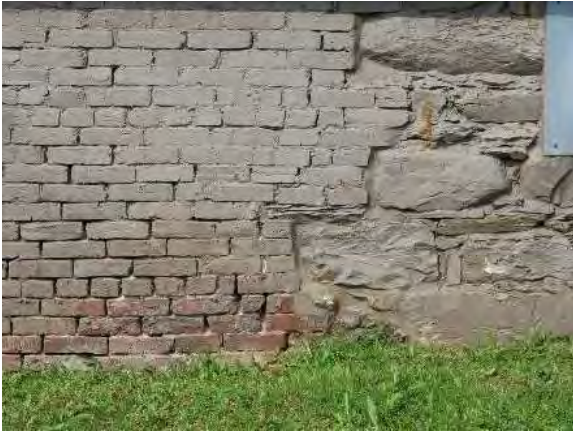
Photo 13: Segment of stone foundation repaired with brick, looking west
