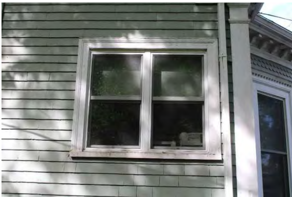
Photo 12: Wood window surrounds and wood sills on a side façade, looking west
