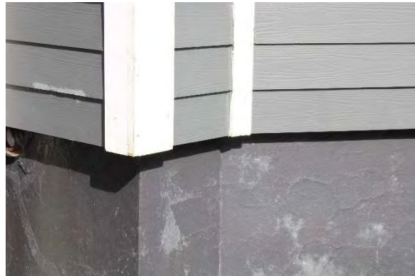
Photo 11: Modern siding and parged and painted foundation from the east façade, looking northwest
