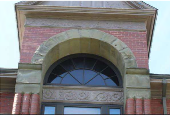
Photo 23: Stone arch and stone decorative panels on the front façade, looking southwest
