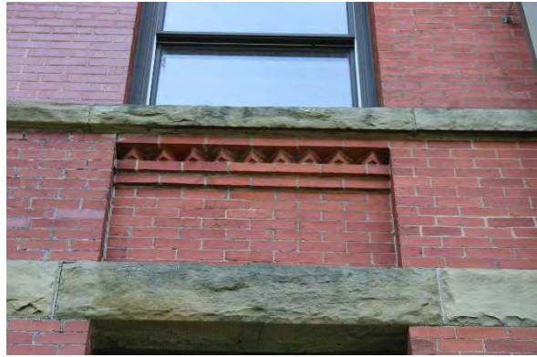
Photo 24: Example on front façade of sawtooth brick work and stone belt courses seen in multiple locations on the structure, looking southwest
