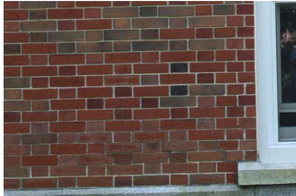
Photo 5: Sample of Flemish bond brick pattern from the north façade, looking southeast
