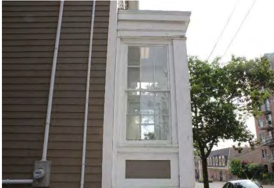
Photo 8: Wood cornice, wood frame windows and wood paneling of porch, looking east
