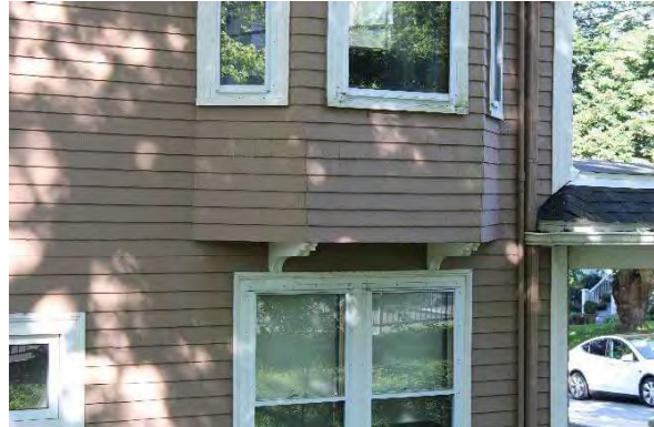
Photo 12: Wood brackets on second storey bay window of east façade, looking west
