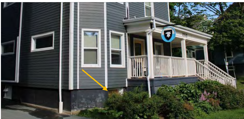
Photo 9: Elevated basement with windows (denoted by arrow) that requires steps for accessing the front entrance, looking northwest
