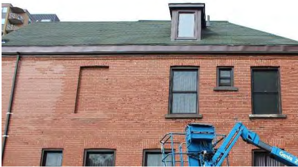
Photo 20: Filled in window and brick repairs on the east façade, looking west
