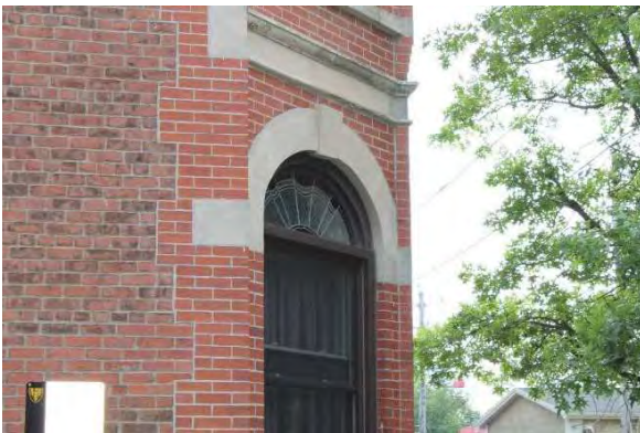
Photo 18: Seam between front façade and west façade, looking east
