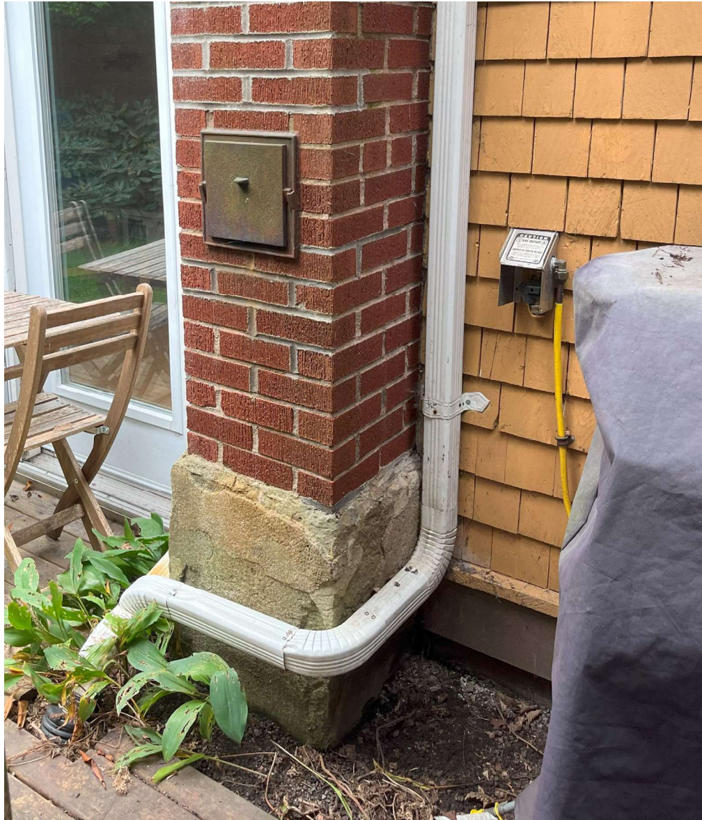
Figure 19: Photograph of rear addition of Porters House with second exterior chimney (Staff visit, September 19 th , 2024)
