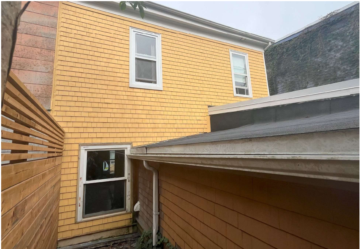
Figure 17: Photograph of Porters House from the west elevation (Staff visit, September 19 th , 2024)
