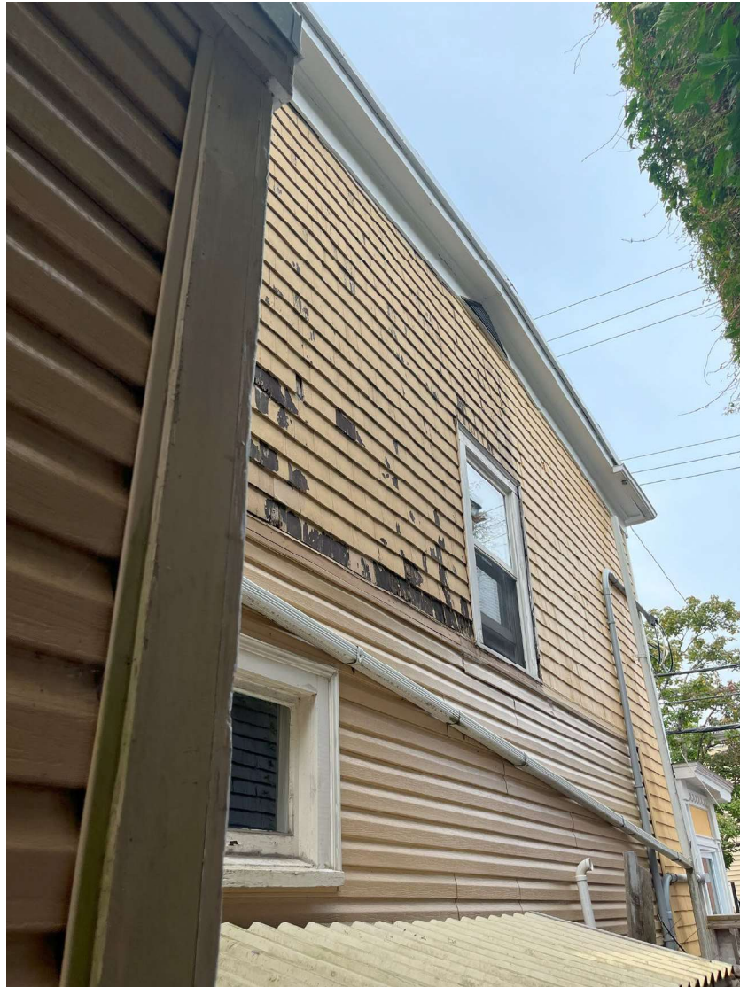
Figure 18: Picture of Porters House from south elevation showing the flat pitch of the roof with projecting verges and portion of house with vinyl siding (Staff visit, September 19 th , 2024)
