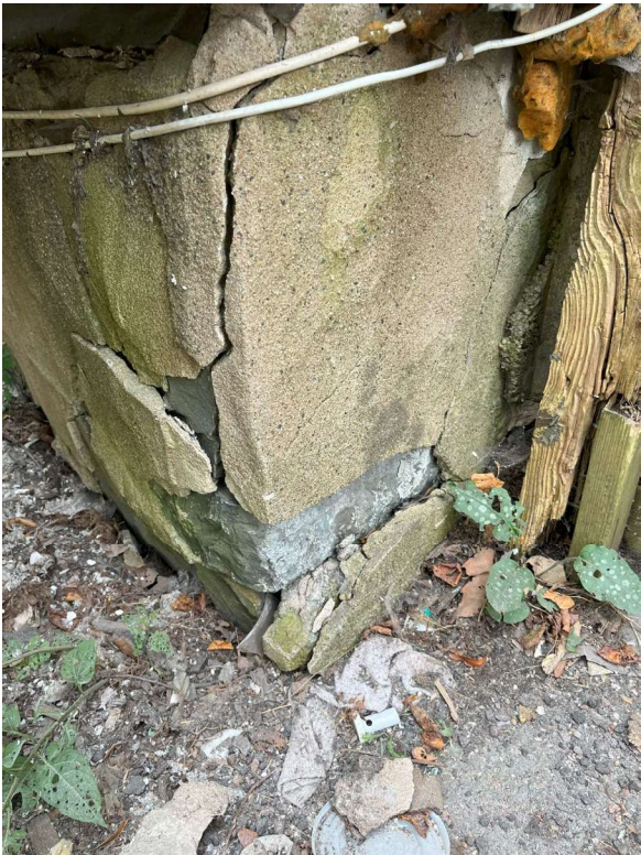
Figure 11: Photograph of corner foundation of 2320 Maynard as viewed from sidewalk (Staff visit, September 19 th , 2024)
