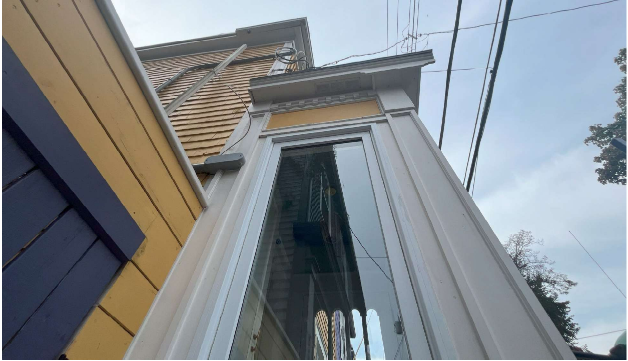
Figure 16: Photograph of Porters House of south elevation of storm porch (Staff visit, September 19 th , 2024)
