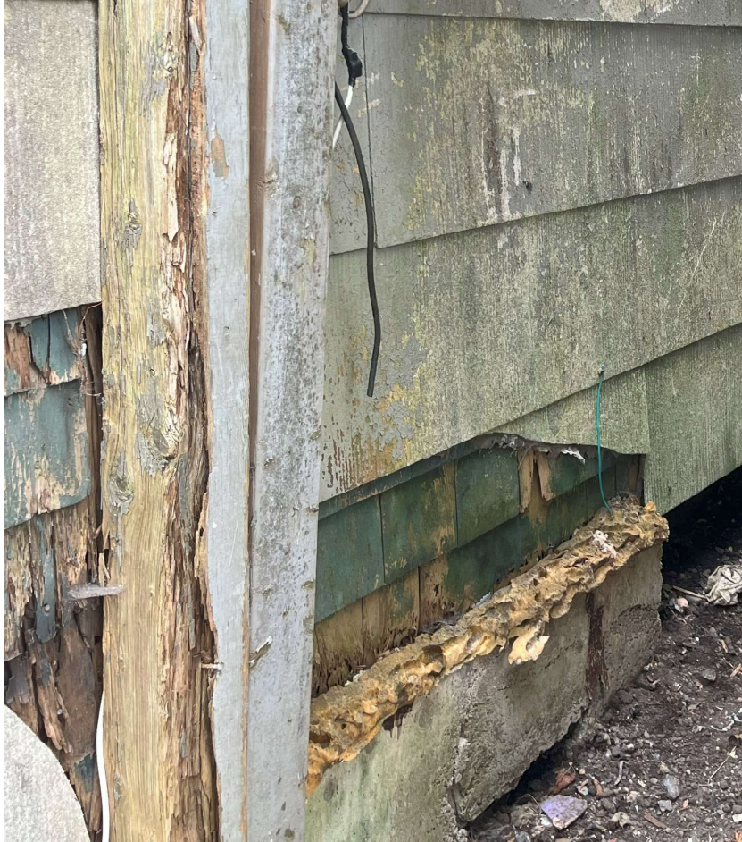
Figure 20: Photograph of siding on north elevation of 2320 Maynard showing underneath new vinyl siding (Staff visit, September 19 th , 2024)
