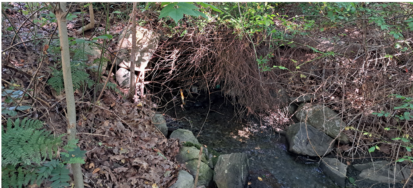
Potential Watercourse surfaces out of stormwater culvert across Mic Mac Boulevard (HRM Planned Growth)
