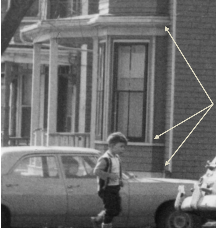
Figure 22: Photograph of first storey bay window and porch in 1967 with wood trim highlighted (Robertson, 1967).
