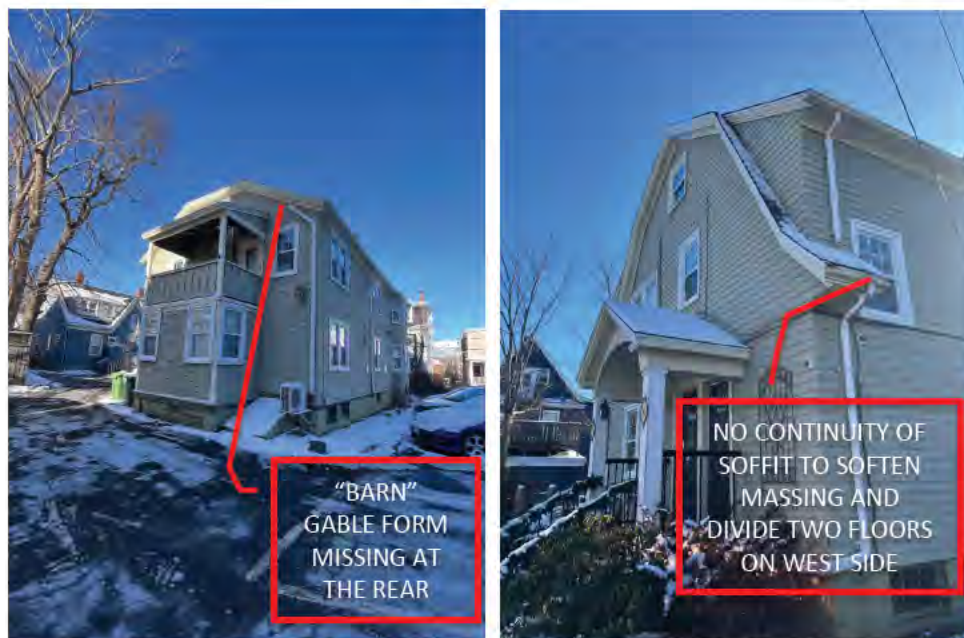
Figure 36c: Front and rear components of 43-45 Dundas Street that detract from the style and overall design of a Dutch Colonial Revival house.
