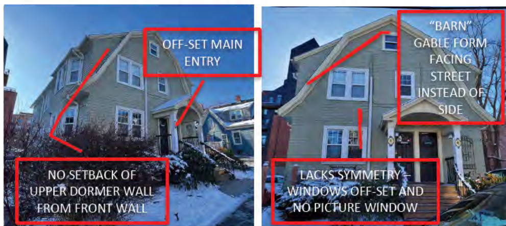
Figure 36a: Front components of 43-45 Dundas Street that detract from the style and overall design of a Dutch Colonial Revival house.
