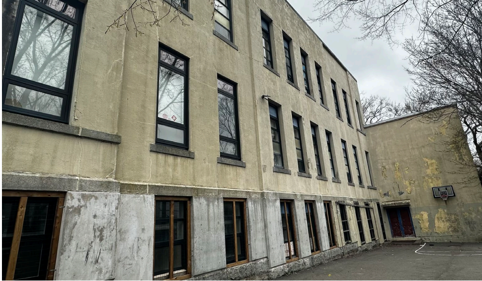
Figure 15: South elevation of the original portion of 5450 Russell Street, and west elevation of rear wing (May 1, 2024)
