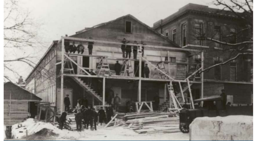
Temporary Dining Hall for Reconstruction Workers after the Halifax Explosion, with 5450 Russell Street to the right
