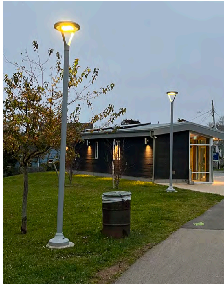
Figure 11: Park pathway lighting in Fort Needham Memorial Park is downward directed, evenly spaced, and connects destinations without gaps in lighting coverage (Cushing, 2023).
